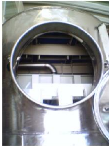
Figure nº 1.5 – CAS+® system's internal components (distributor and demister) photo.
