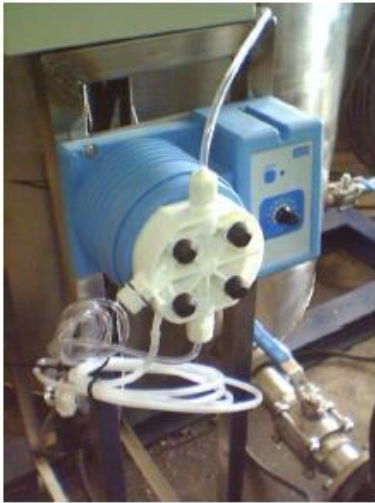
Figure nº 1.4 – CAS+® system's dosing pump photo.
